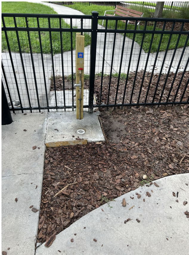
Existing wash station with mulch, erosion, and poor drainage
